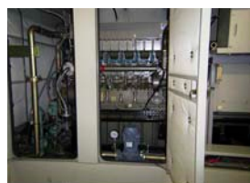
Cogeneration system (gas-fired generator)
