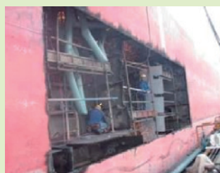
The Pacific Bravery's starboard hull after removal of damaged panel
