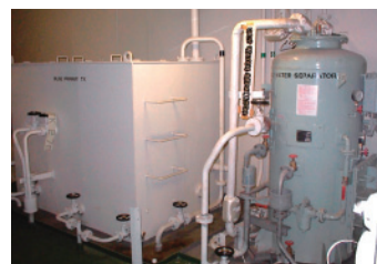
Bilge primary tank (left) Bilge separator (right)
